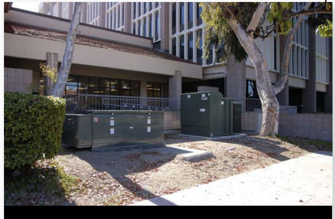
Davidson Library Vista switchgear and 2500-kVA padmount transformer.
