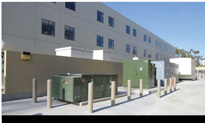
Electrical service area for advanced engineering/research building.
