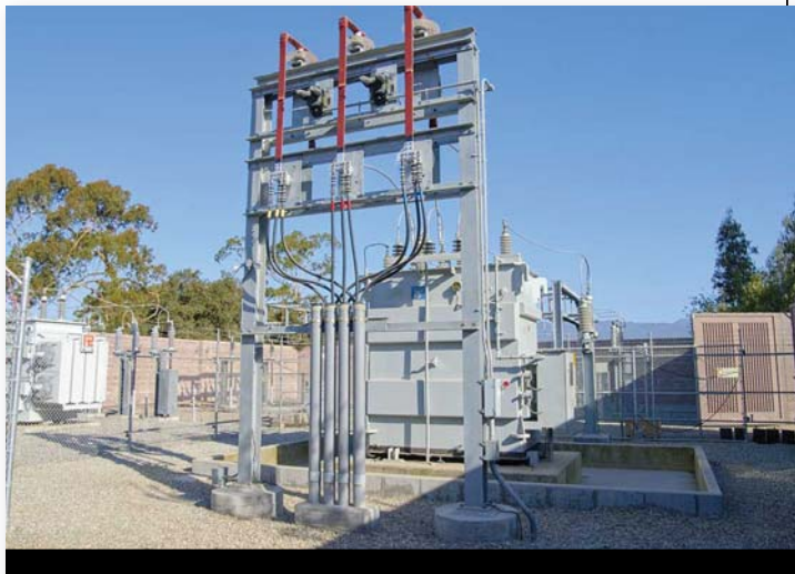
The 12.47-kV side of the new University of California, Santa Barbara-owned 20-MVA 66/12.47-kV substation.
