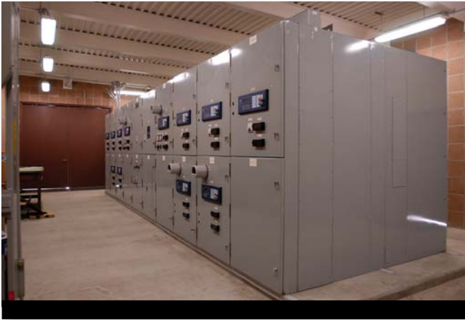
New switchgear building with new indoor vacuum circuit breaker and metal-clad switchgear.
